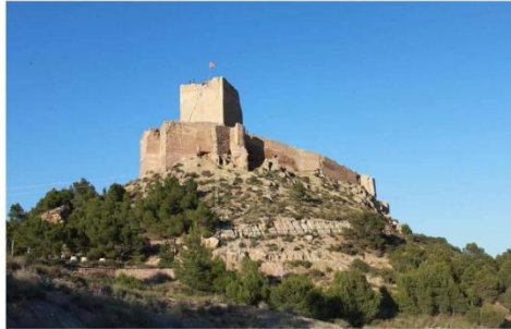
Shear crack onto the castle tower – sliding toward north direction
